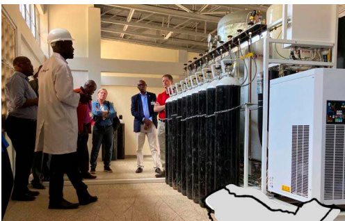
The oxygen plant at Maua Methodist Hospital.
